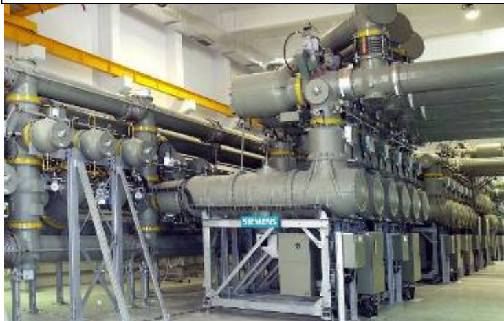
Gas-Insulated Substations (GIS)
