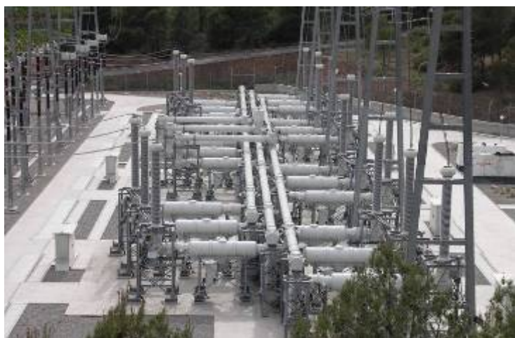
Highly-Integrated Substations (HIS)
