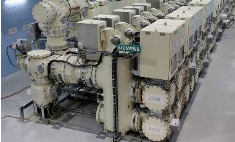
Gas-Insulated Switchgear (GIS)
