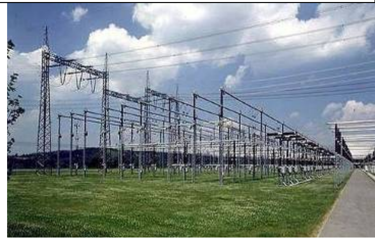
Air-Insulated Substations (AIS)
