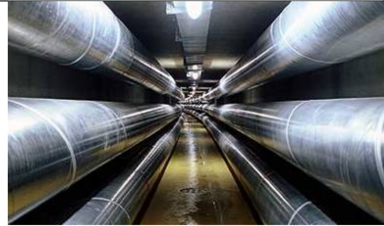
Gas-Insulated Lines (GIL)
