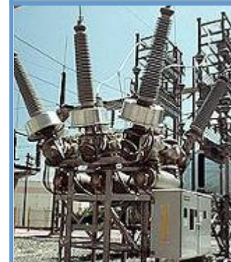
Dead Tank Switchgear Bay
